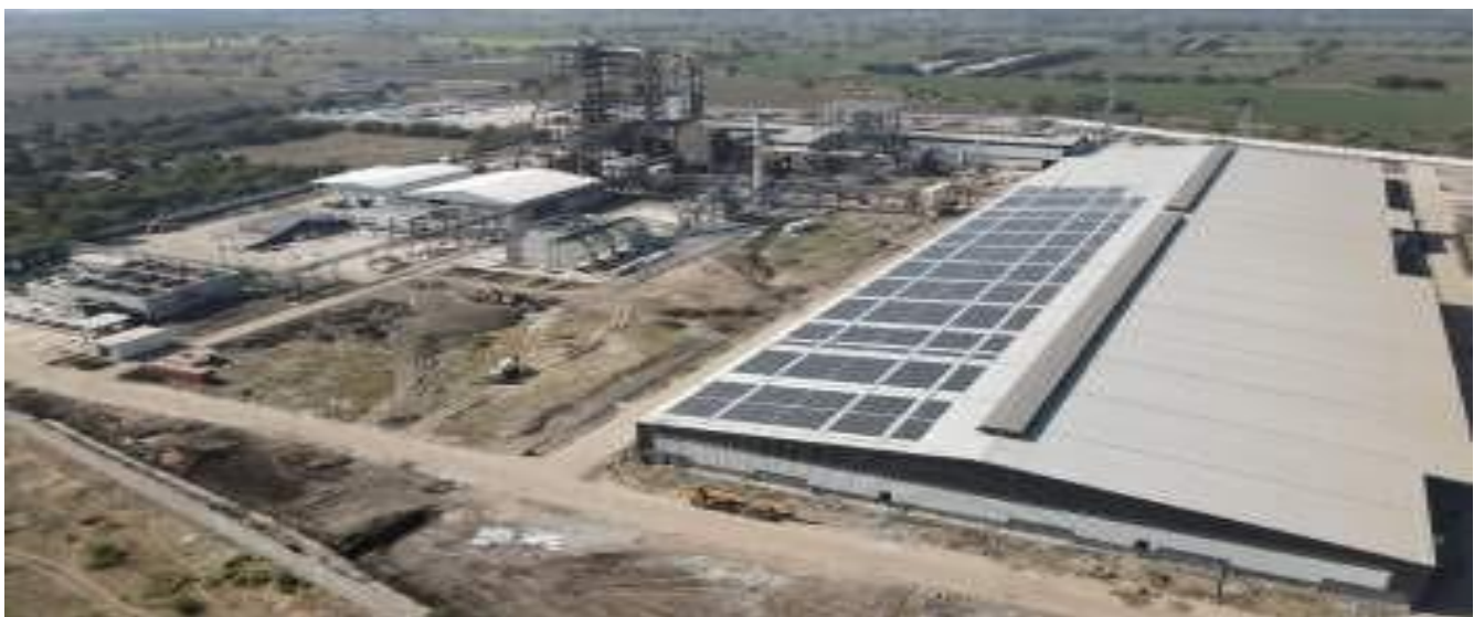
Rooftop Solar Panels at Greenfield MDF Board Manufacturing Facility at Vadodara, Gujarat
